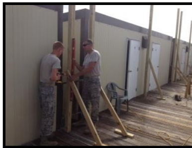
SMSgt Emehizer and SrA Hagler ensure columns are level for an overhead shelter.
