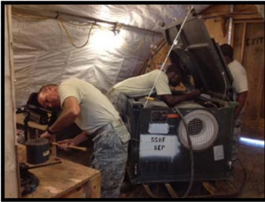
MSgt Baldwin, SrA Barnett and SrA Mathews work on Environmental Control Units
